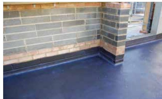
For continuity of waterproofing, TT Vapour Membrane is lapped up to DPC level
