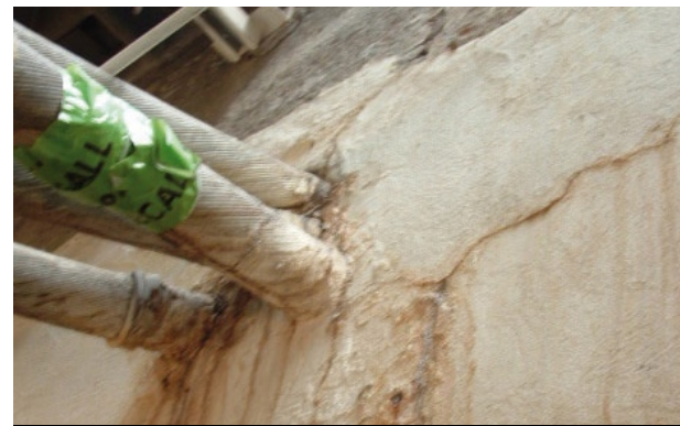
Render cracked and debonded in light wells
