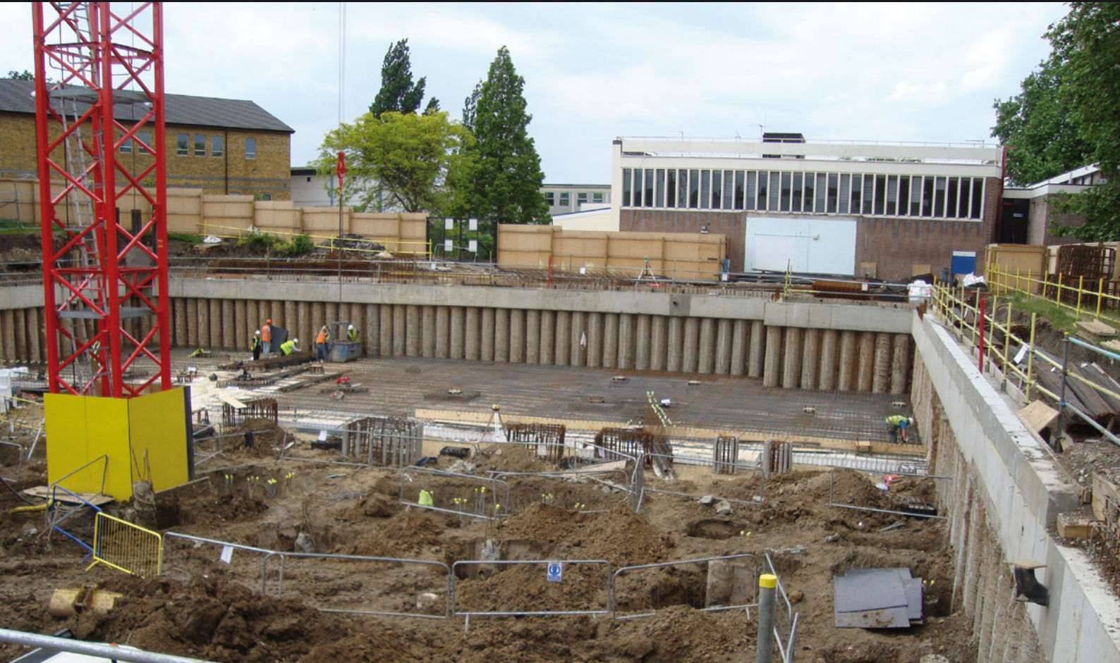
The first of three pours in the construction of the watertight concrete floor slab
